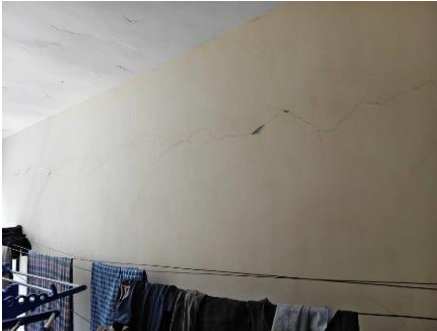
Slab concrete spalling off due to corrosion of steel and wall cracks at wall Beam junction.
