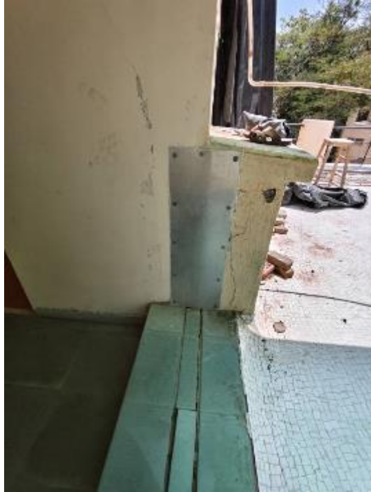
Damages and cracks in Roof water proofing & Expansion joint
