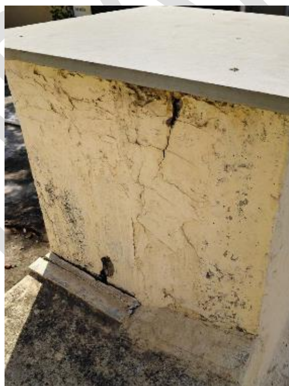
Expansion Joint damage
