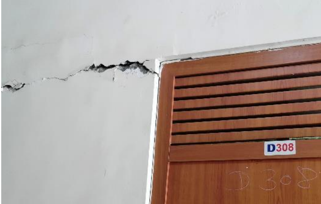
Non-structural Cracks at top floor of Hostel Buildings.
