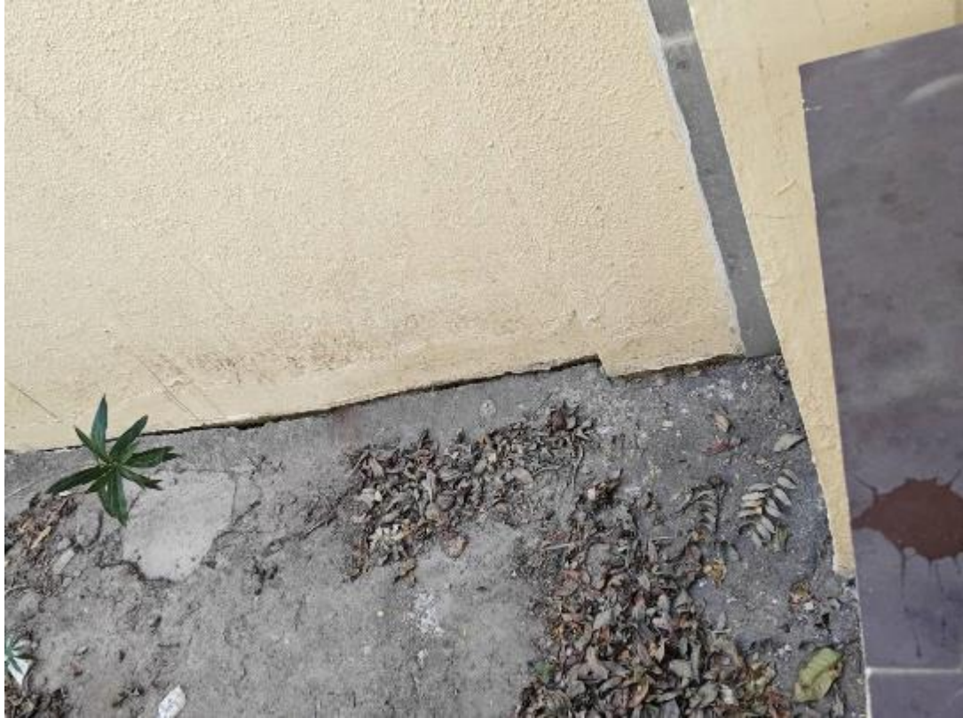
Plinth protection settlement
