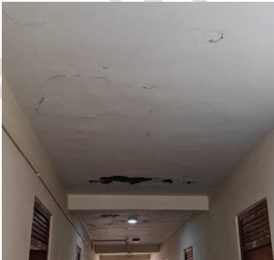
Slab Concrete pill off due to corrosion of steel
