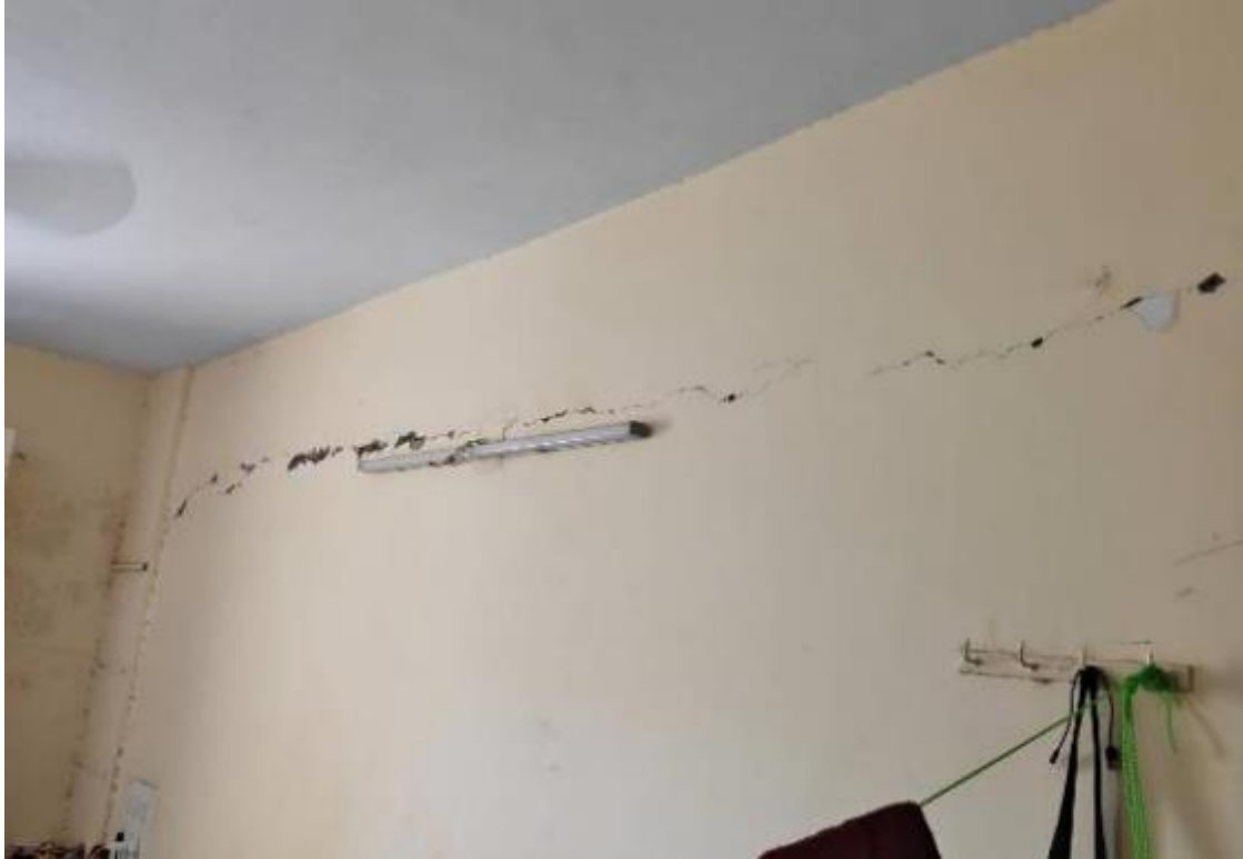
Non-structural Cracks at top floor of Hostel Buildings.
