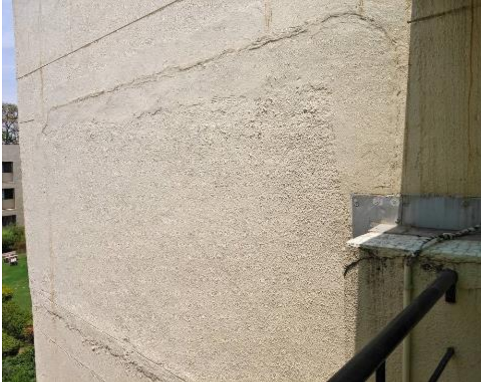
Previously repaired of wall plaster and structure.
