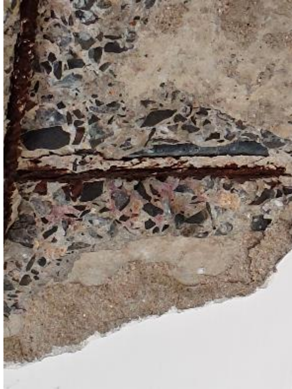
Carbonation at slab Level
