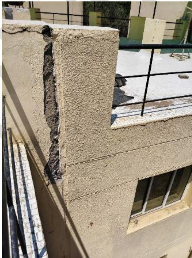
Damages and cracks in water proofing & Expansion joint
