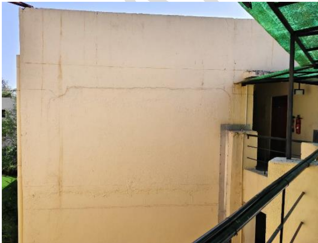
Non-structural Cracks at top floor of Hostel Buildings.
