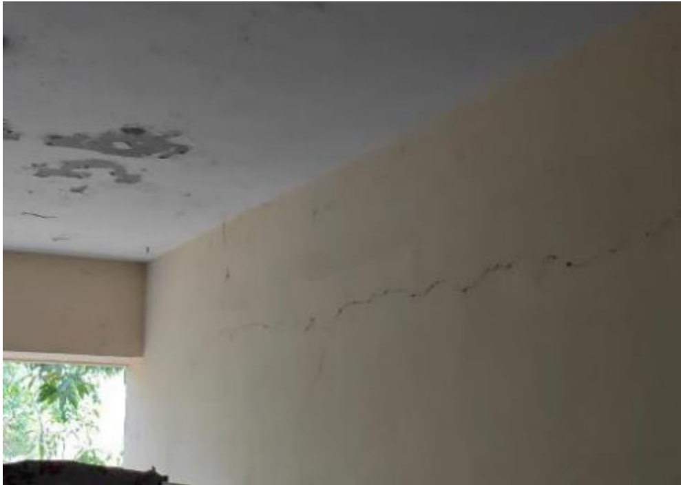
Dampness and corrosion in Slab & Crack below Beam.
