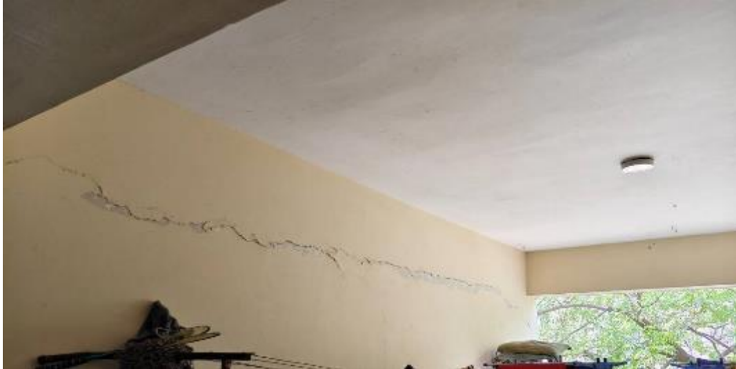
Non-structural Cracks in open chowk and outer walls of rooms
