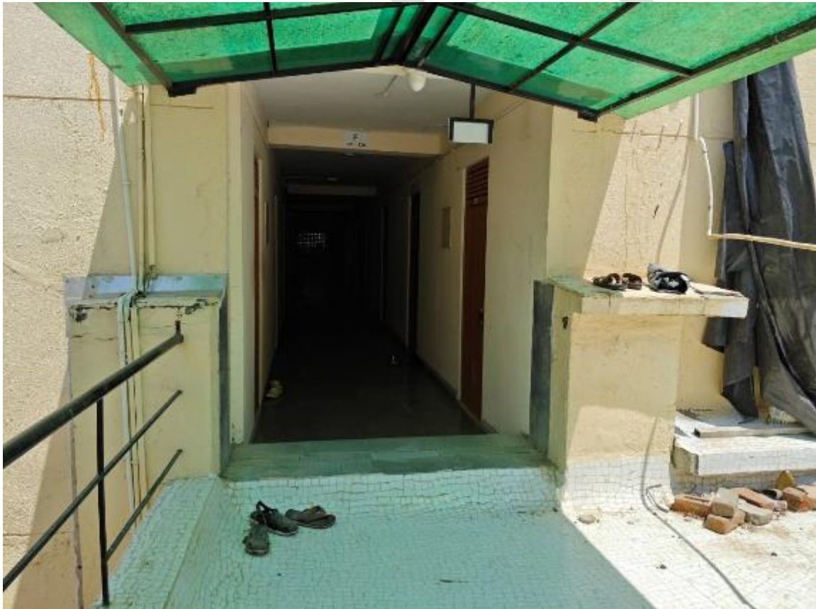
Damages and cracks in Expansion joint water proofing.
