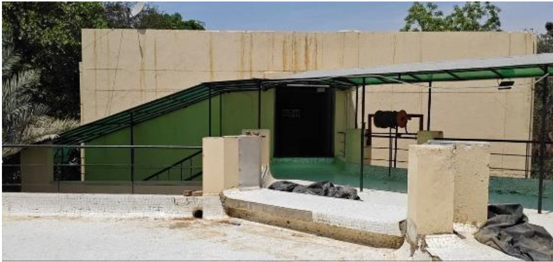
Damages and cracks in Roof water proofing & Expansion joint
