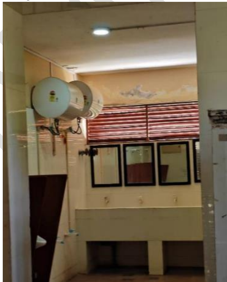
Dampness and Leakage in Washroom area.
