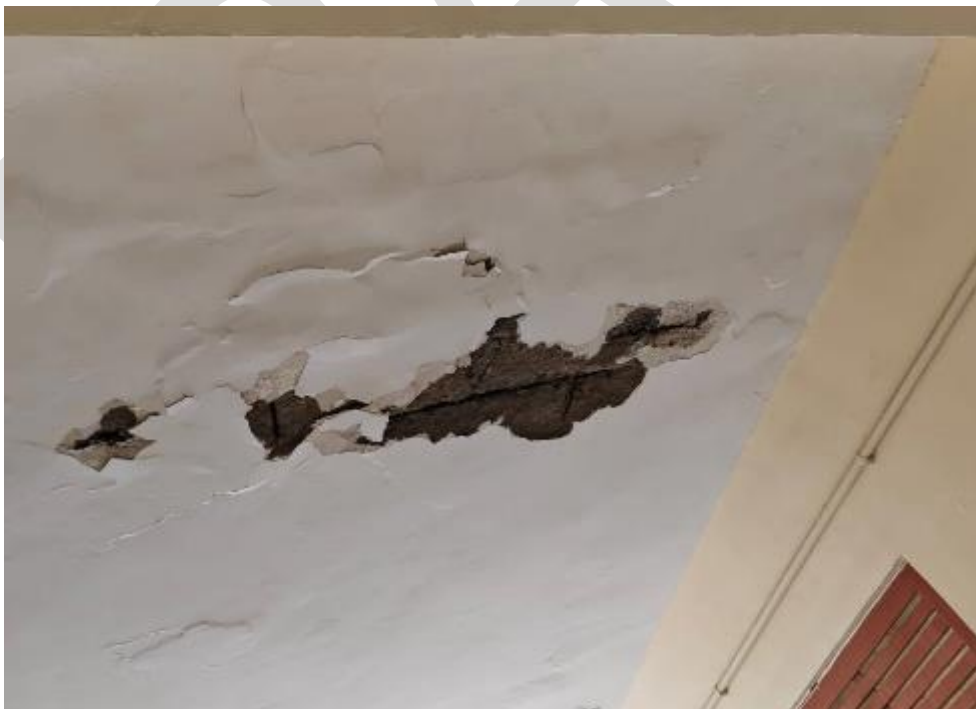
Slab Concrete spilling off due to corrosion of steel
